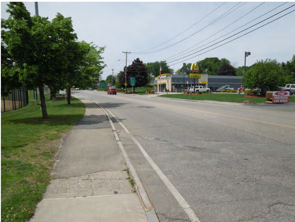
AUBURN STREET – SIDEWALK, GRANITE CURBING AND PAVEMENT CONDITIONS
