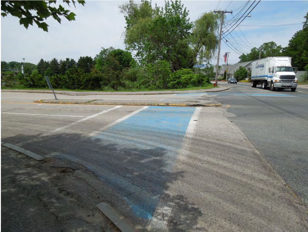
BROTHERTON WAY CROSSWALK (ADA ACCESSIBILITY ISSUE)
