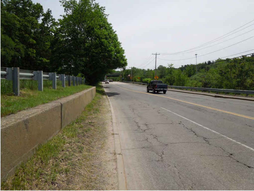
AUBURN STREET (LOOKING SOUTH) PAVEMENT CONDITION/LACK OF SIDEWALK
