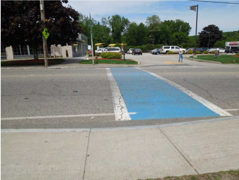
AUBURN STREET CROSSWALK SOUTH OF HIGH SCHOOL ENTRANCE (ADA ACCESSIBILITY ISSUE)
