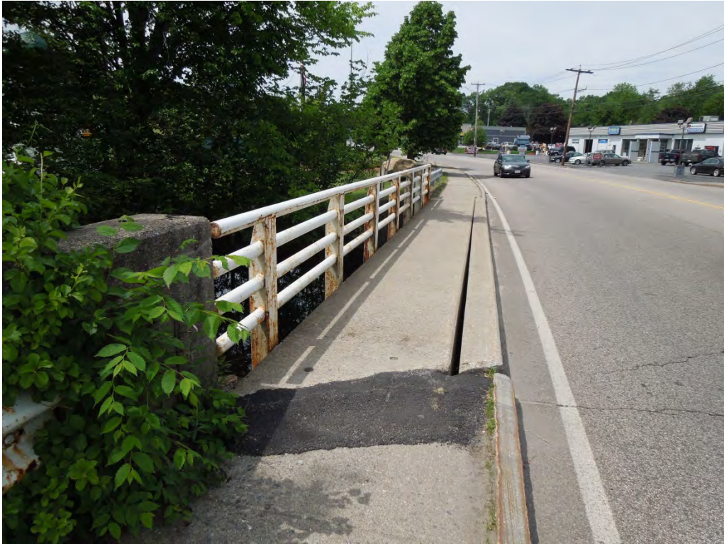
AUBURN STREET BRIDGE OVER RAMSHORN BROOK (ADA ACCESSIBILITY ISSUE)
