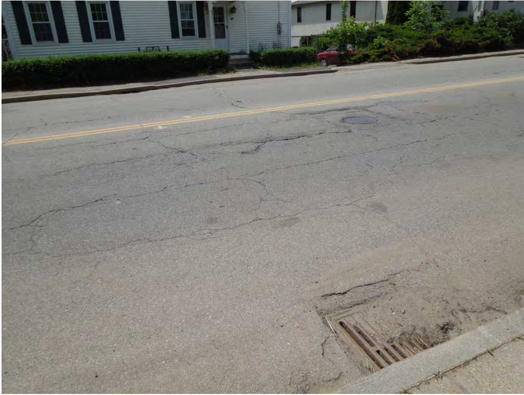
AUBURN STREET – DRAINAGE CONDITIONS
