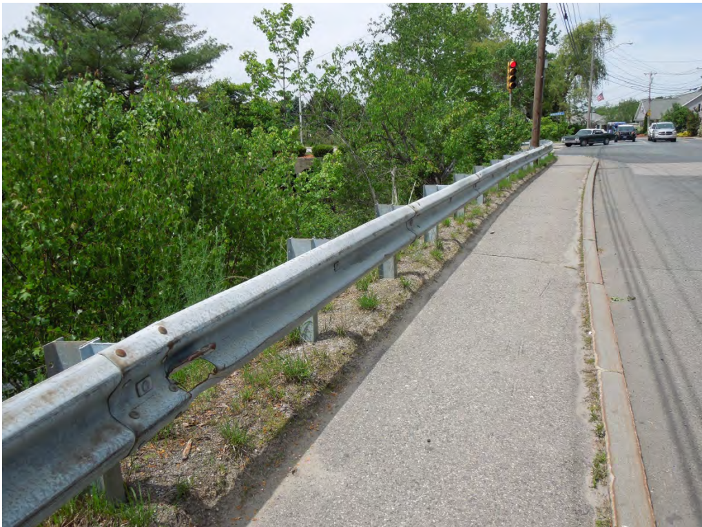
AUBURN STREET AT BROTHERTON WAY INTERSECTION – GUARDRAIL CONDITION
