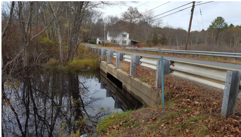
Undersized culvert at Willow Brook and George Street, Mendon
