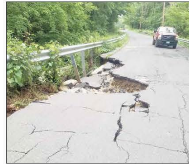
Brook Road also experienced severe damage from last July's flooding. Photo Courtesy of James McKeon
