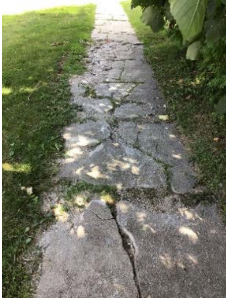
Figure 1: Main Street Sidewalk in Poor Condition. Source: CMMPO.
