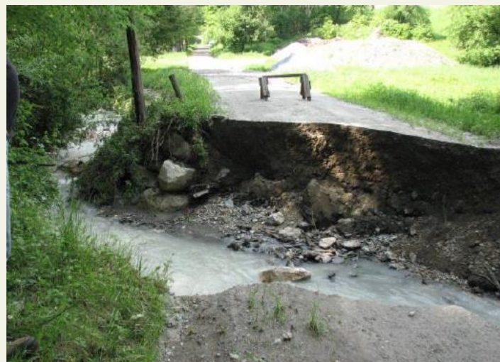
Figure 15: Example of a Failed Culvert [12]
