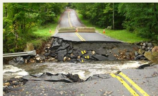
Figure 16: Example of a Failed Culvert [1]
