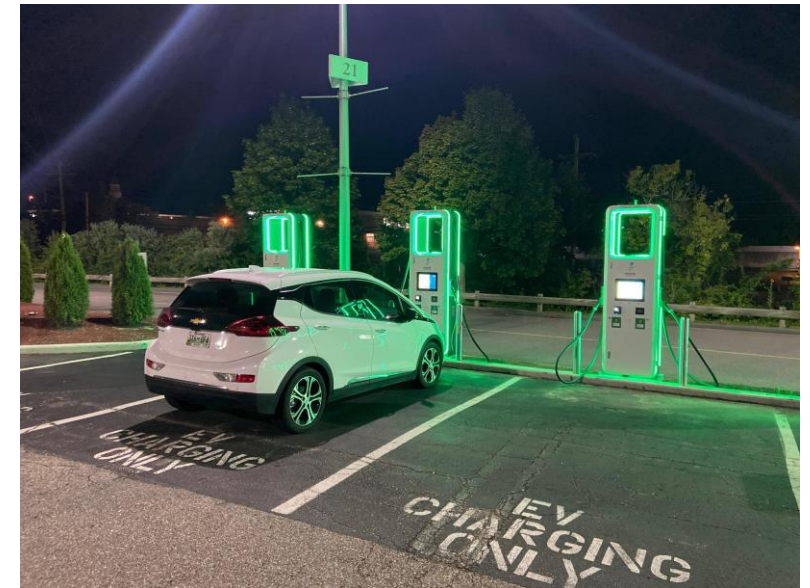
PlugShare Chargers at Auburn Mall
