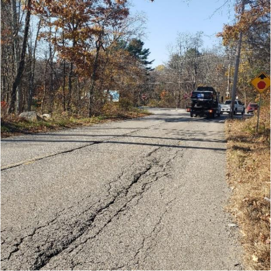
Figure 23: Pavement on Cedar Hill Road in Marlborough
