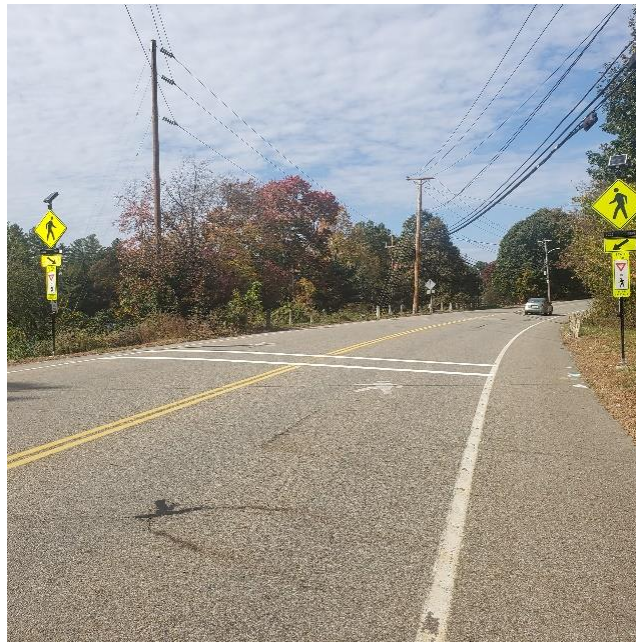
Figure 18: Bartlett Street Crosswalk with RRFB Signal
