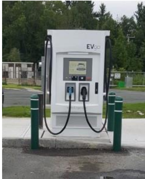
Figure III-20: MassDOT Electric Vehicle Charging Station
